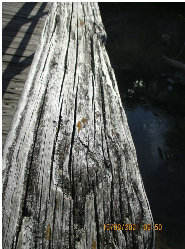
Figure 14 : South Bridge Barrier Top Face_Evidence of Severe Weathering
