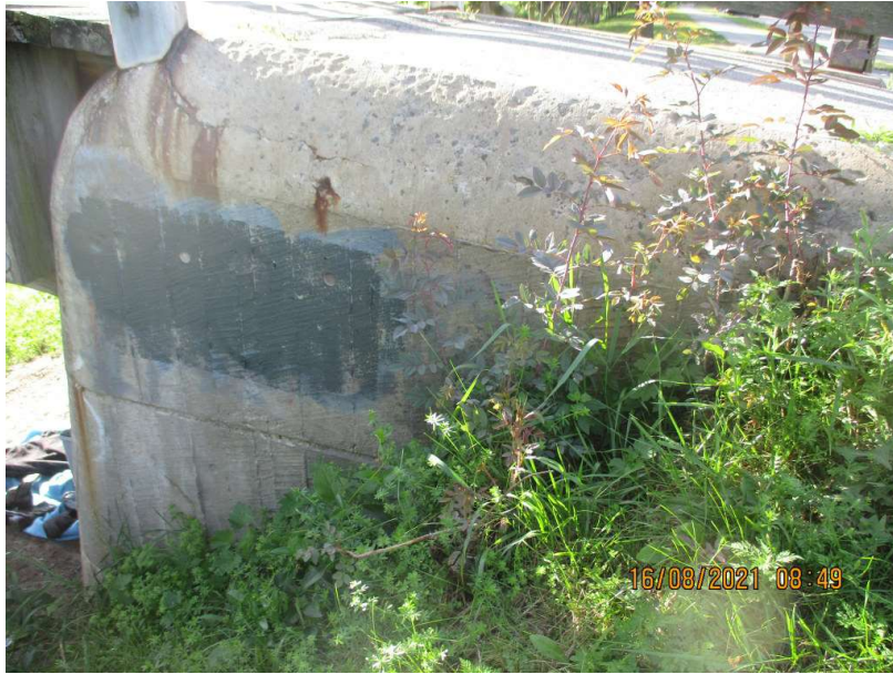
Figure 9 : NW Wingwall_Evidence of Wide Cracks & Rust Stain around Barrier Connection to Wingwall
