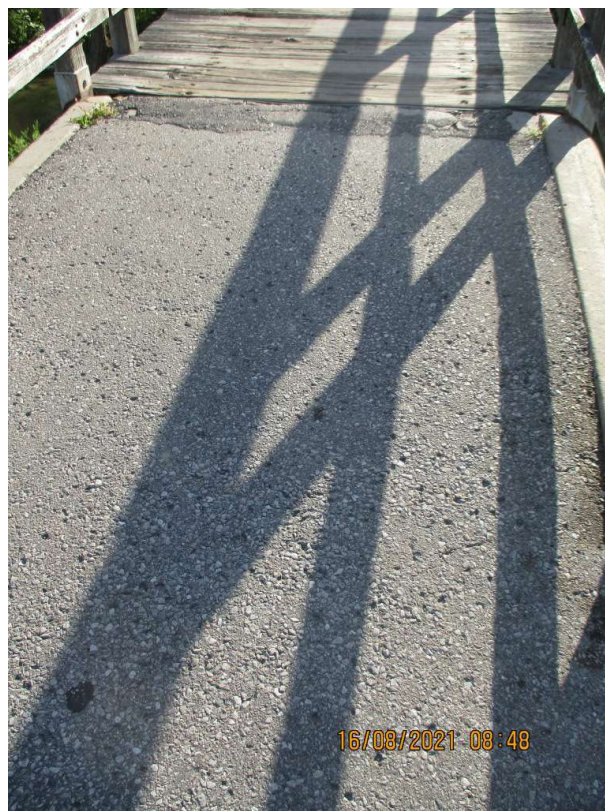
Figure 6 : Asphalt Wearing Surface Condition over West Approach (Typ.)
