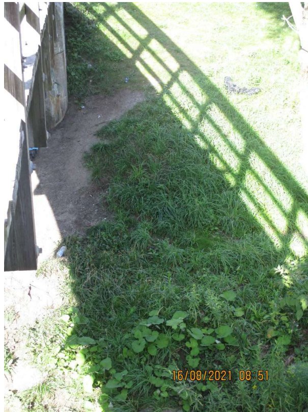
Figure 18 : NW Embankment_Evidence of Medium Erosion
