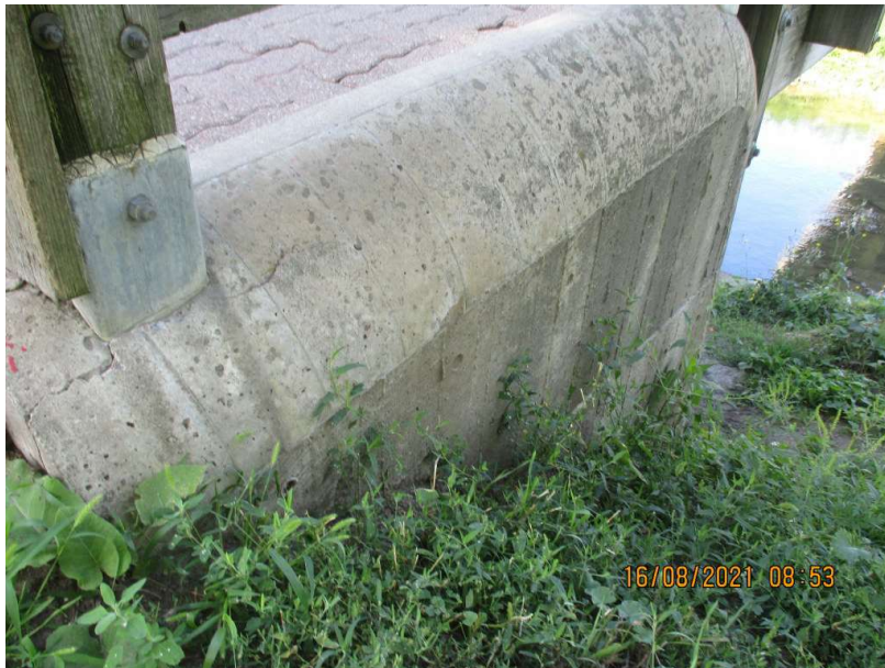
Figure 10 : NE Wingwall_Evidence of Wide Cracks around Barrier Connection
