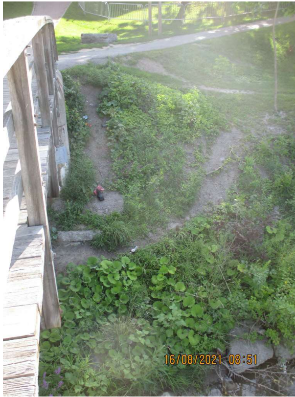
Figure 21 : SE Embankment_Evidence of Medium Erosion
