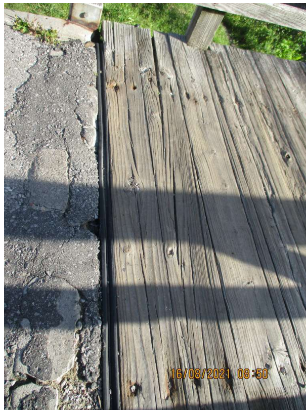
Figure 12 : West Bridge End Condition (Typ.)_Evidence of Spall & Wide Cracks on Exposed Surface of Ballast Wall
