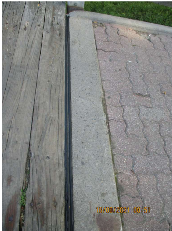
Figure 5 : East Bridge End Condition (Typ.)_Evidence of Medium to Wide Map Cracking & Rust Stain on Ballast Wall
