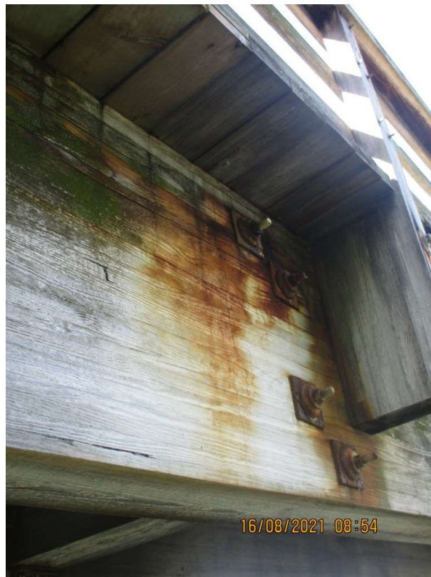
Figure 28 : Post Tensioning Rod Ends_Evidence of Medium to Severe Corrosion
