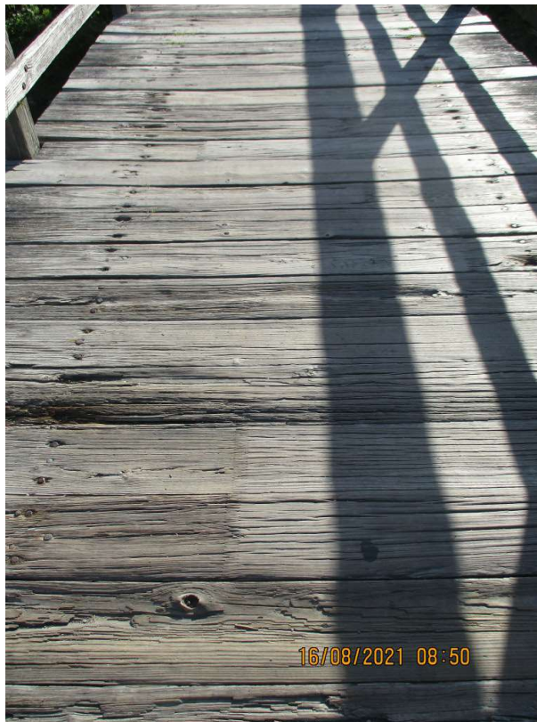
Figure 13 : Deck Top Condition (Typ.)_Evidence of Severe Weathering and Wear & Tear
