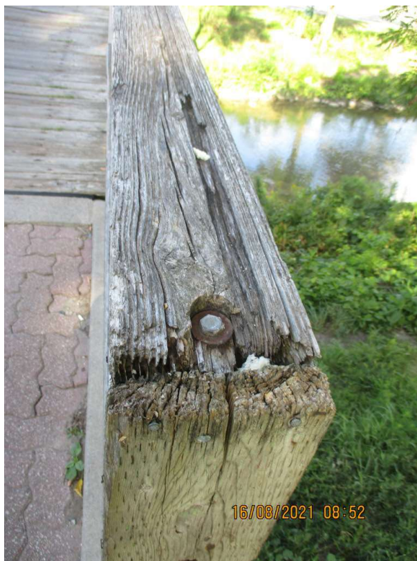
Figure 24 : NE Coener of Barrier_Evidence of Severe Rot
