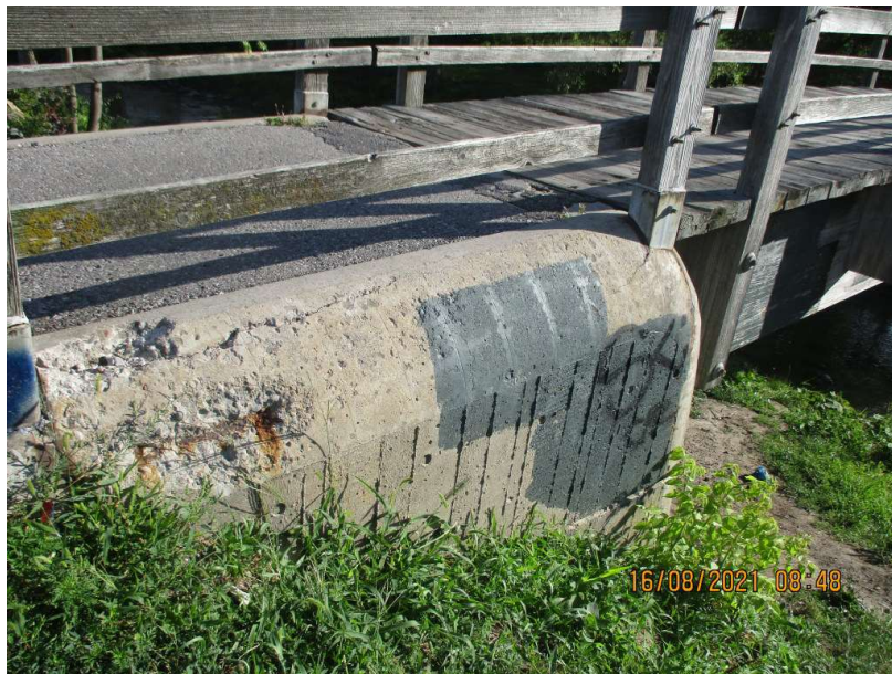
Figure 11 : SW Wingwall_Evidence of Medium Spall, Wide Longitudinal Crack & Rust Stain
