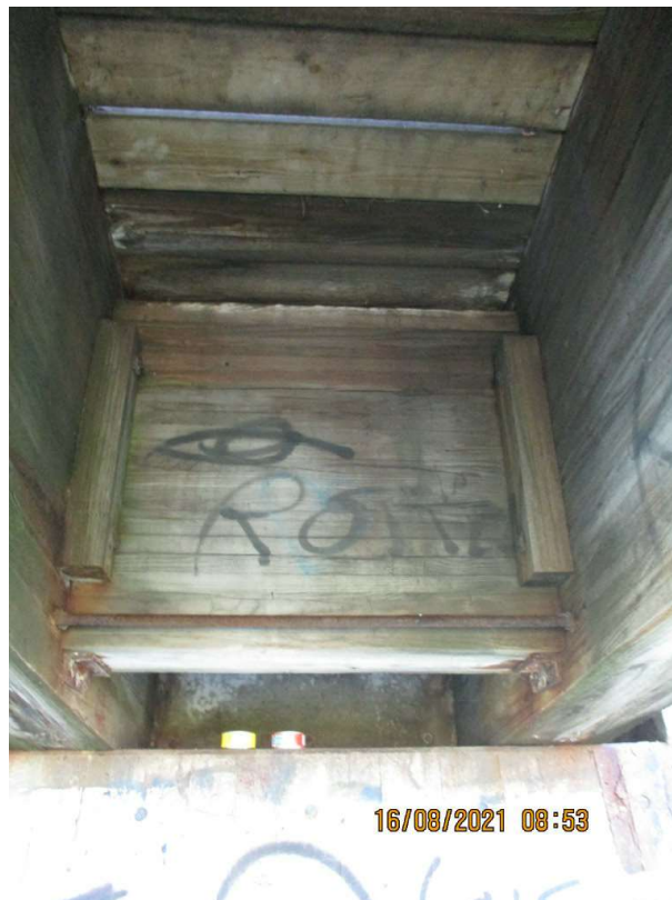
Figure 26 : Timber Diaphragm (Typ.)_ Evidence of Severe Corrosion on Connections
