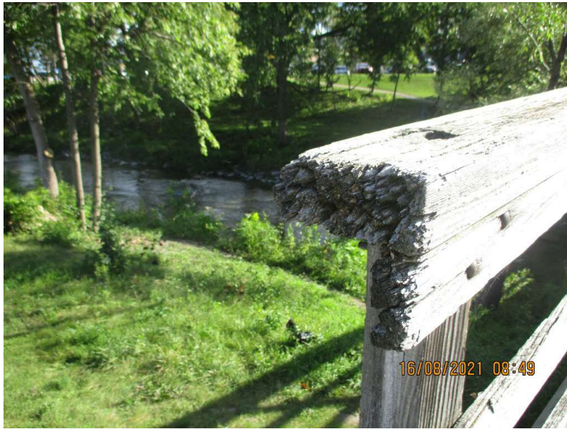
Figure 31 : Approach Barrier_Evidence of Medium Rot
