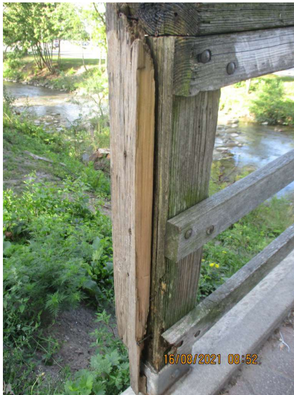
Figure 23 : SE Corner of Barrier_Evidence of Section Loss
