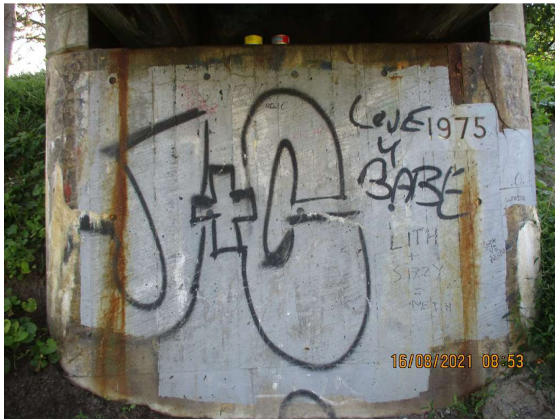
Figure 25 : East Abutment (Typ.)_ Evidence of Wide Transverse Cracks
