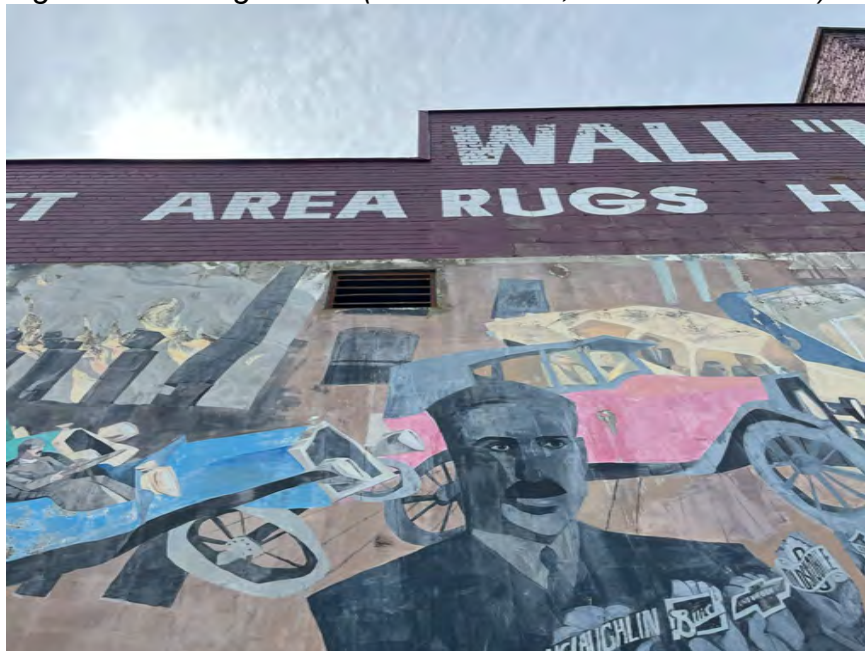
Figure 1: "Driving Force" (Rudolf Stussi, 22 Athol St. East) – Cracks, chips and streaks
