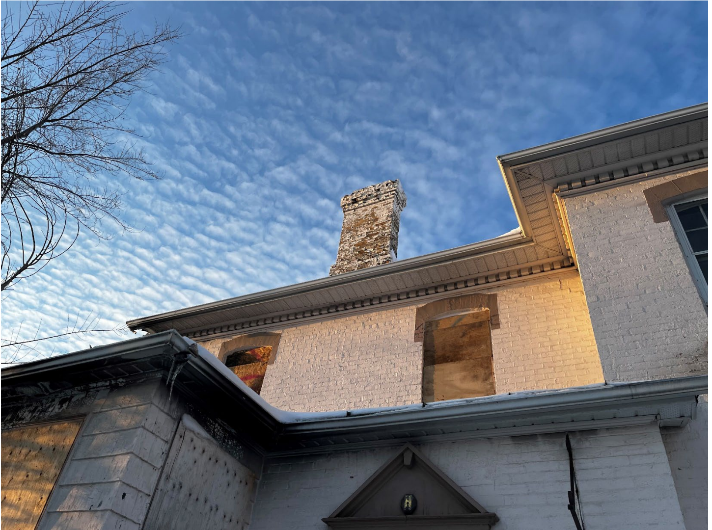
Figure 8 - Deteriorating chimney with potential for restoration
