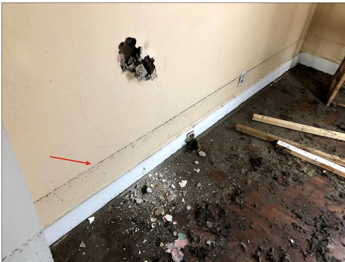
Figure 8: View of water staining line throughout main level and smoke impacted wall finishes in northeast bedroom (Sample S-4)
