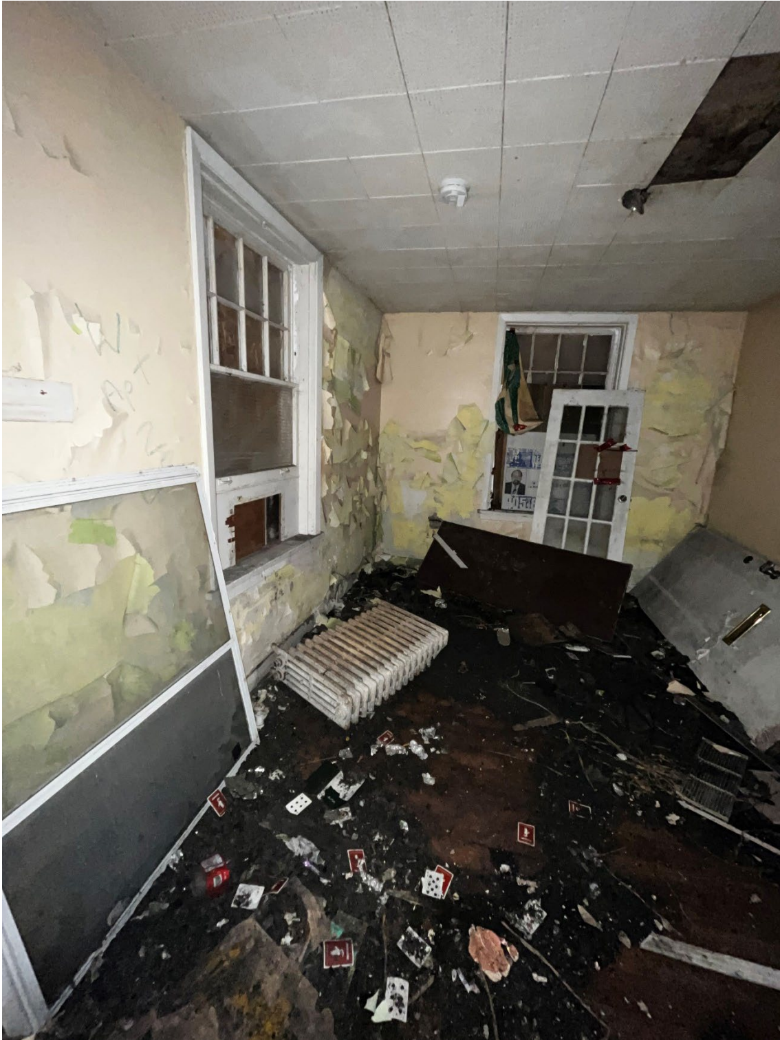
Figure 14 - Showing significant damage
