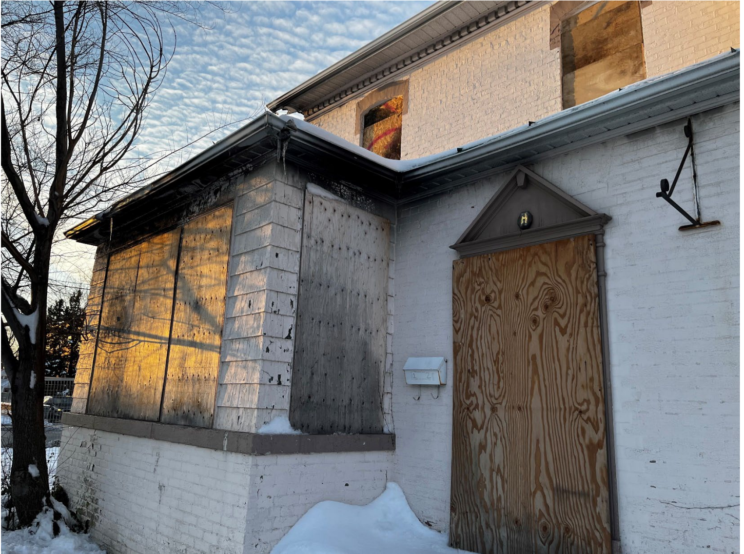
Figure 7 - Fire damage shown around the sunroom
