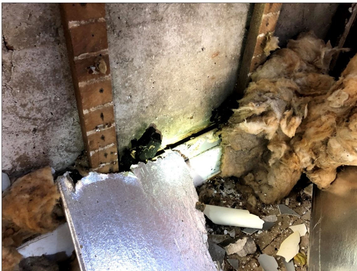
Figure 14: View of smoke impacted perimeter wall cavity in northeast bedroom (Sample S-5) on second level
