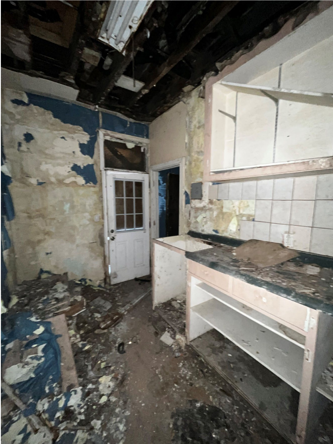
Figure 19 - Showing significant damage.
