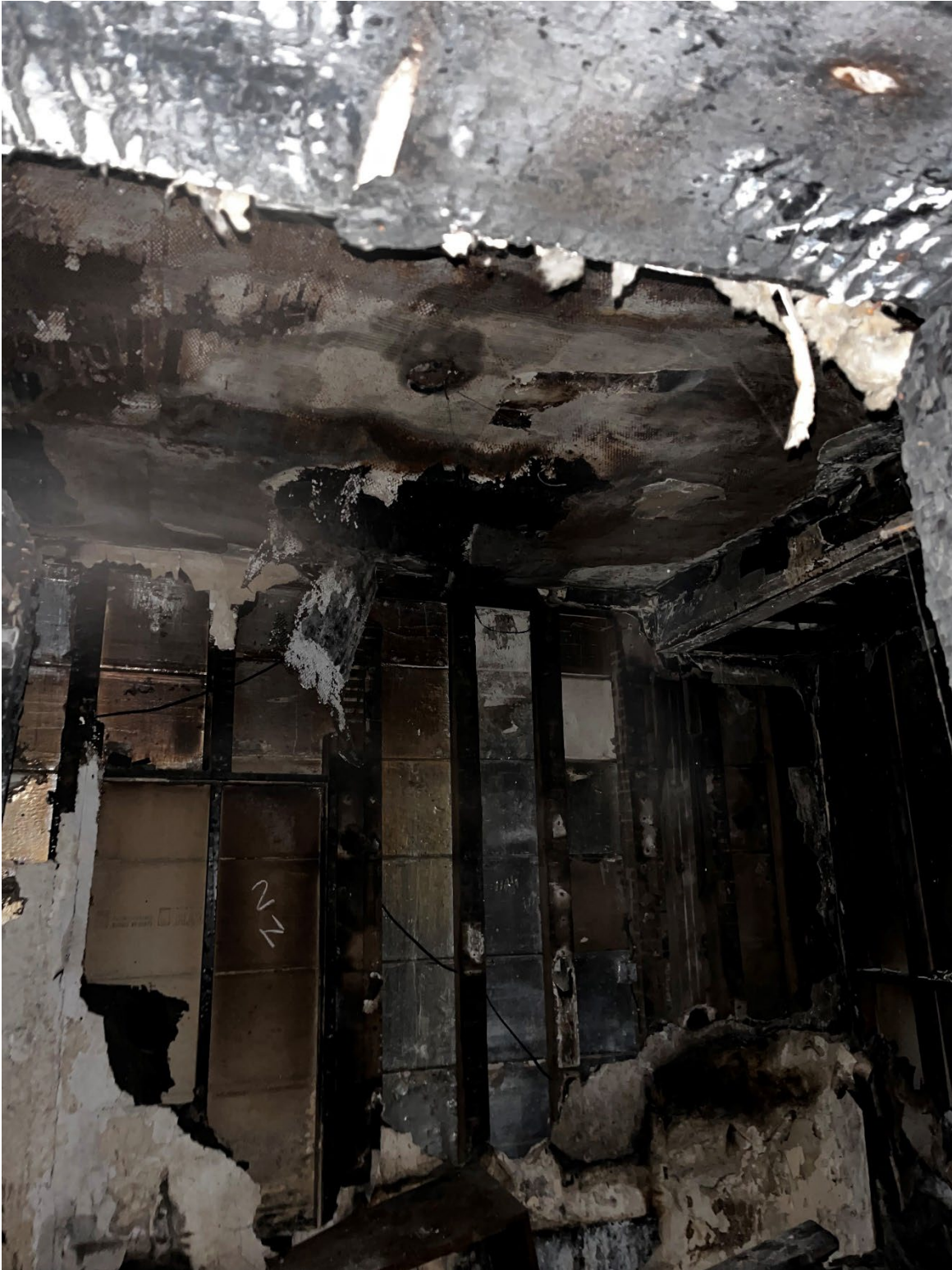
Figure 30 - Showing extent of fire damage, interior black from fire and burn.
