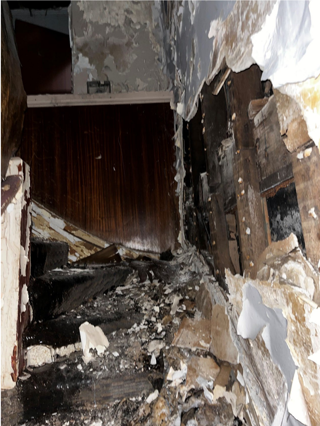
Figure 22 - Showing significant damage where fire spread through wall.
