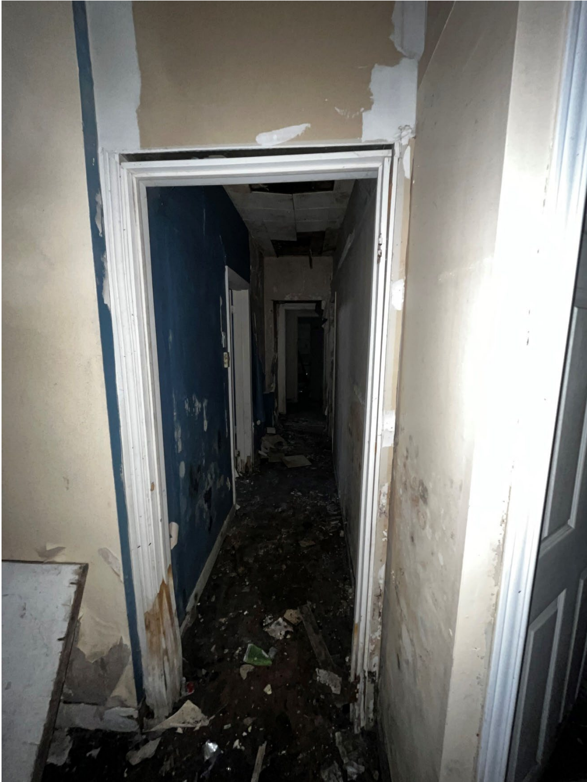
Figure 15 - Showing significant damage
