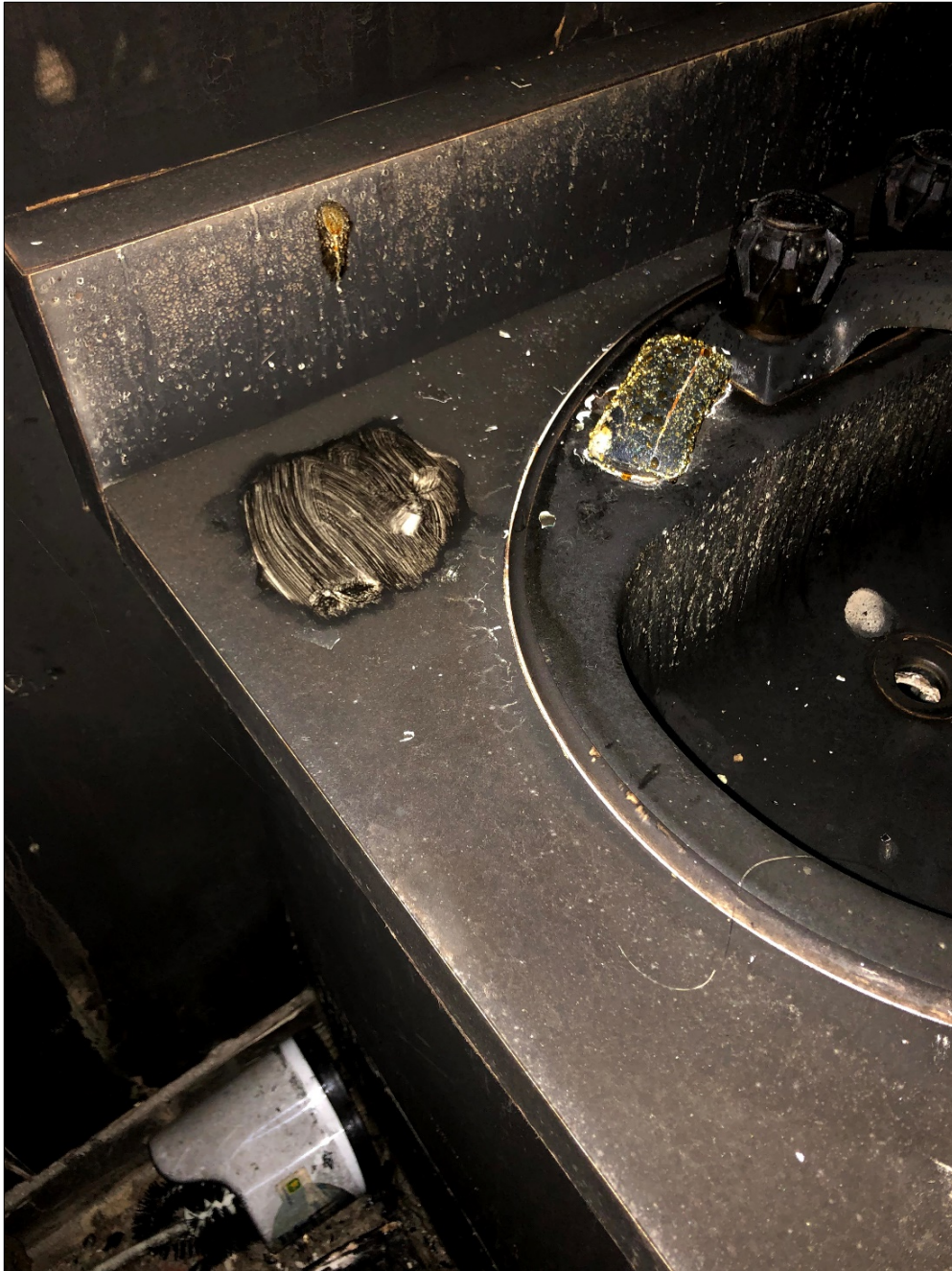
Figure 13: View of smoke impacted vanity in main level east washroom (Sample S-3)
