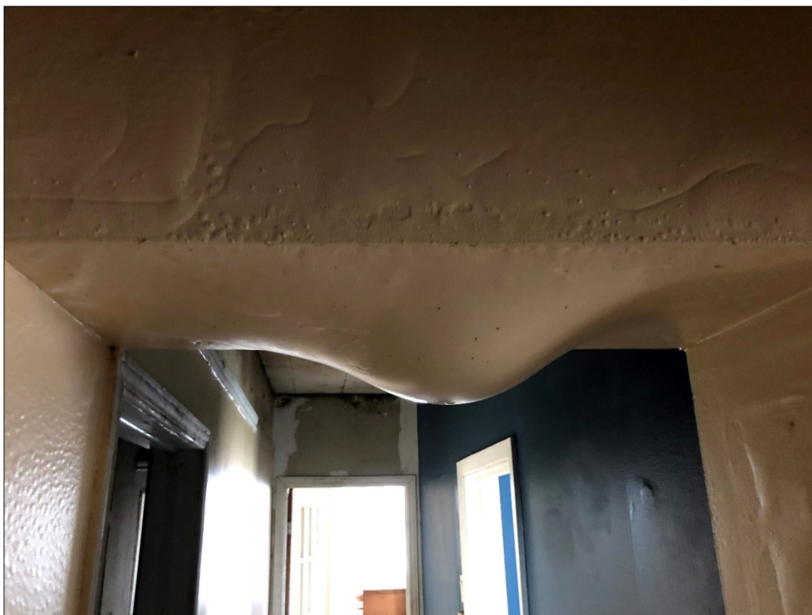
Figure 5: View of water bubble trapped in door header
