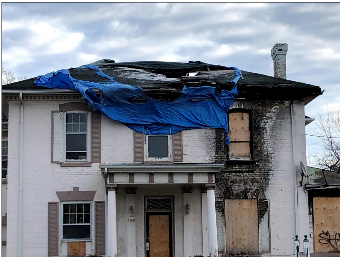
Figure 1: View of front exterior of subject house and roof consumed by fire
