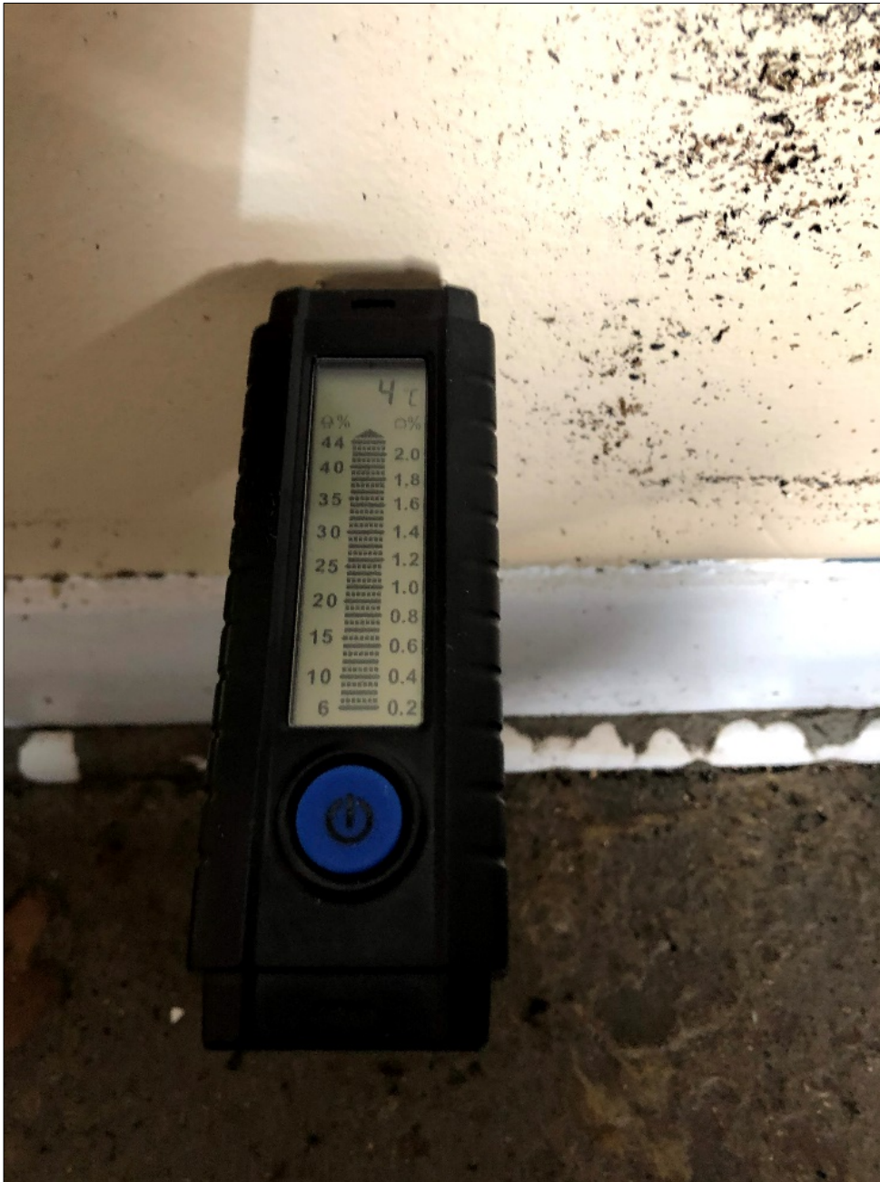
Figure 6: View of moisture meter confirming elevated moisture readings from wall finishes
