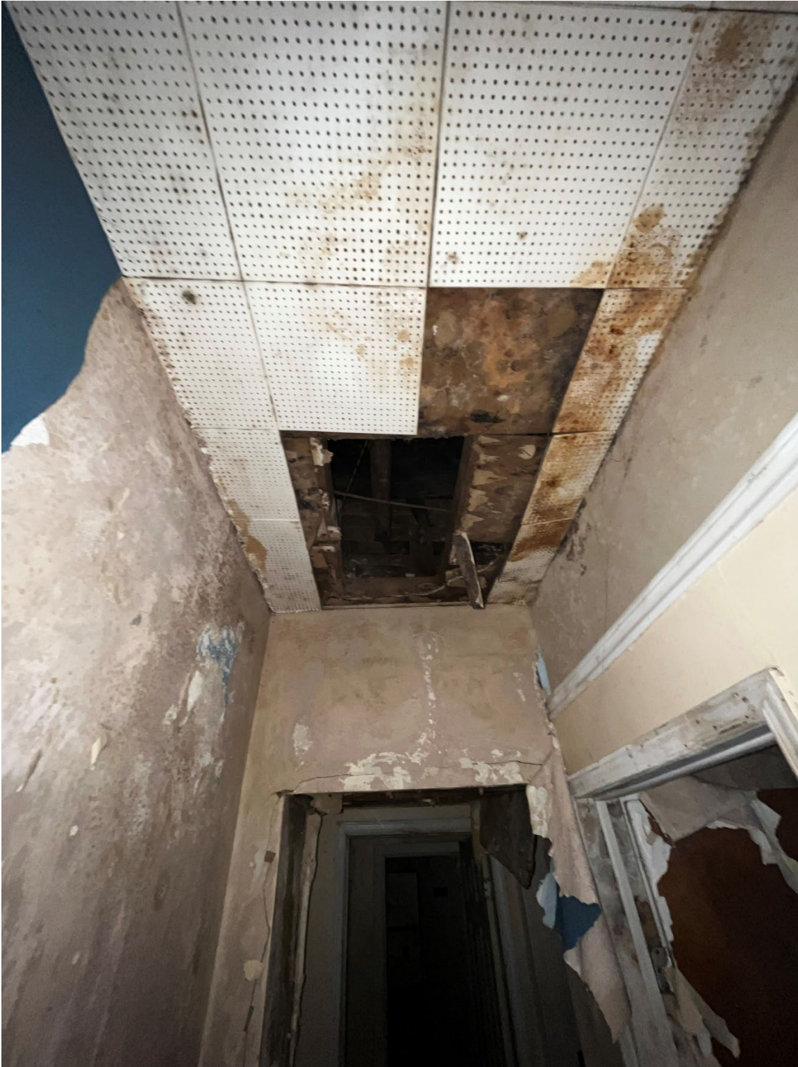
Figure 17 - Showing significant damage.
