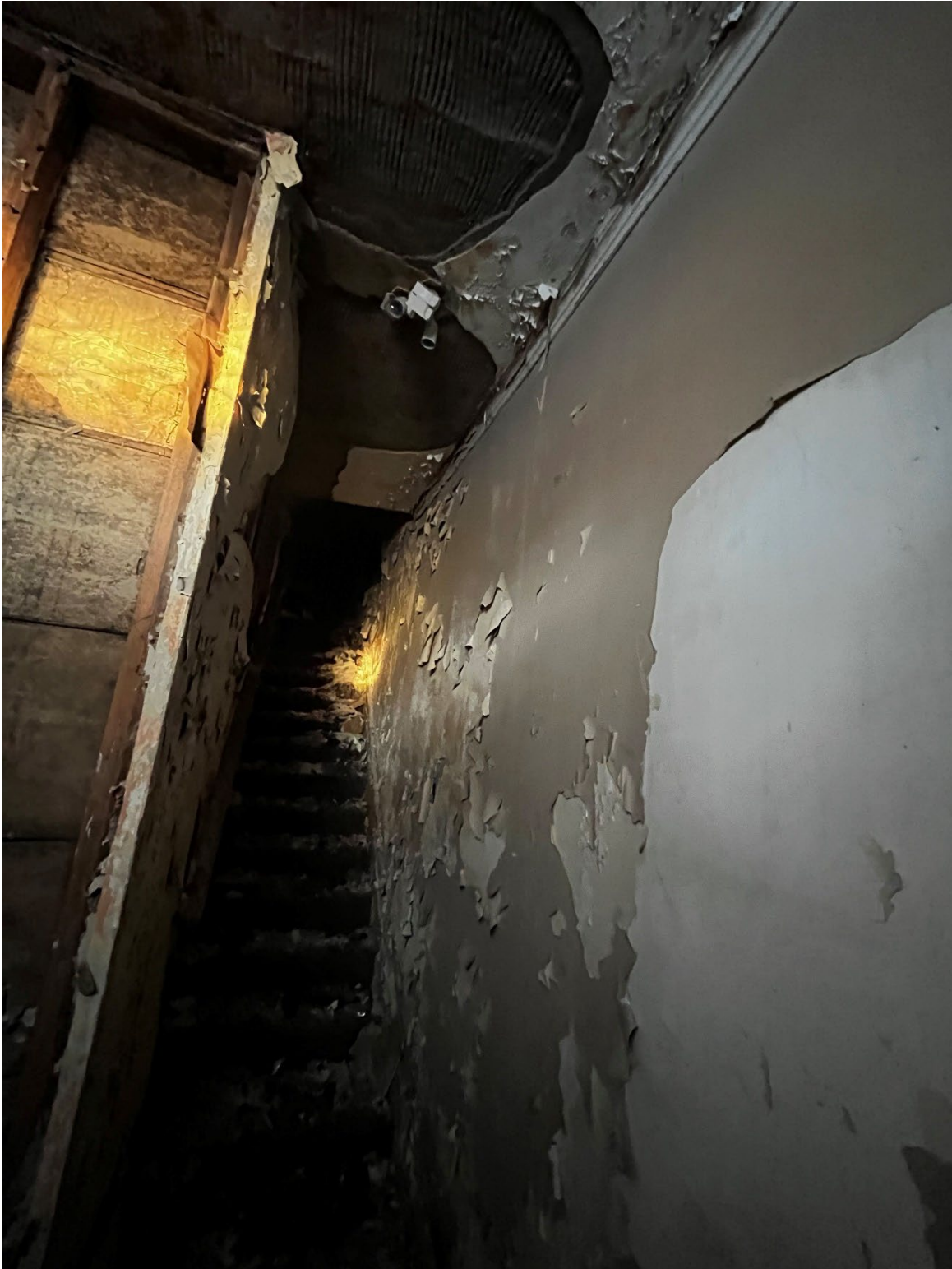
Figure 13 - Staircase showing significant damage.
