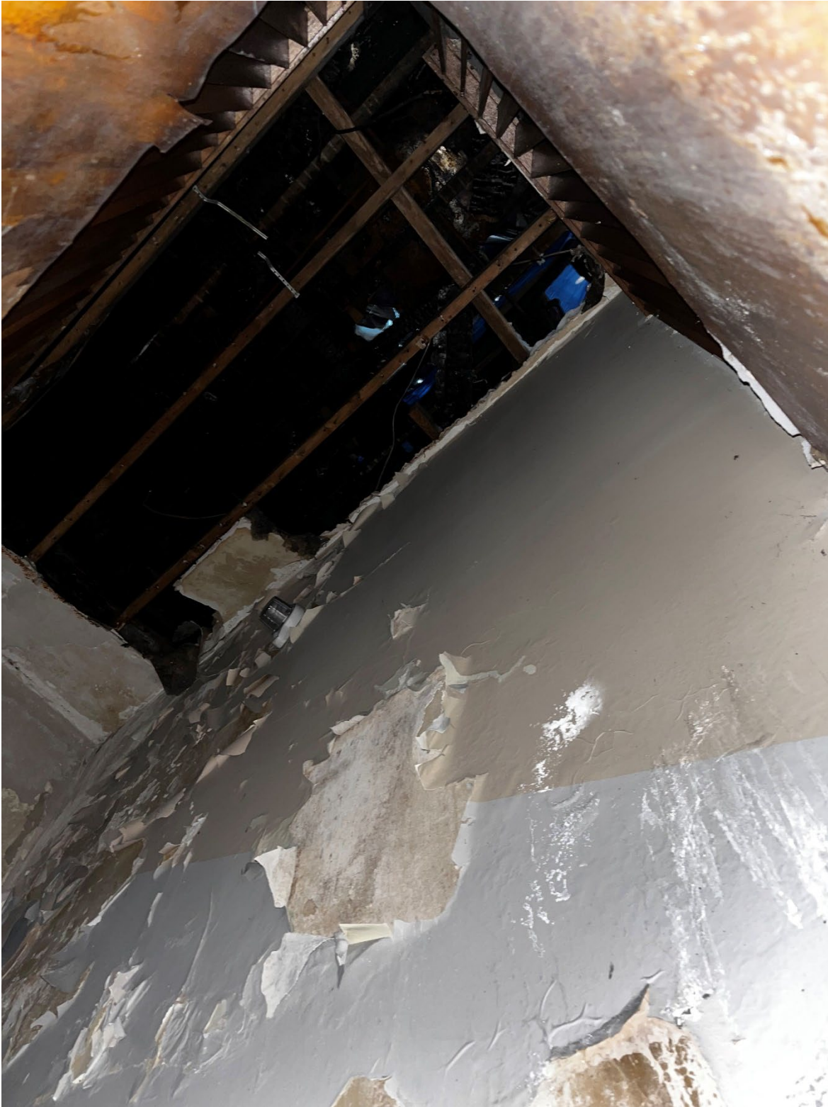
Figure 23 - Showing significant damage where fire caused structural failing of roof.
