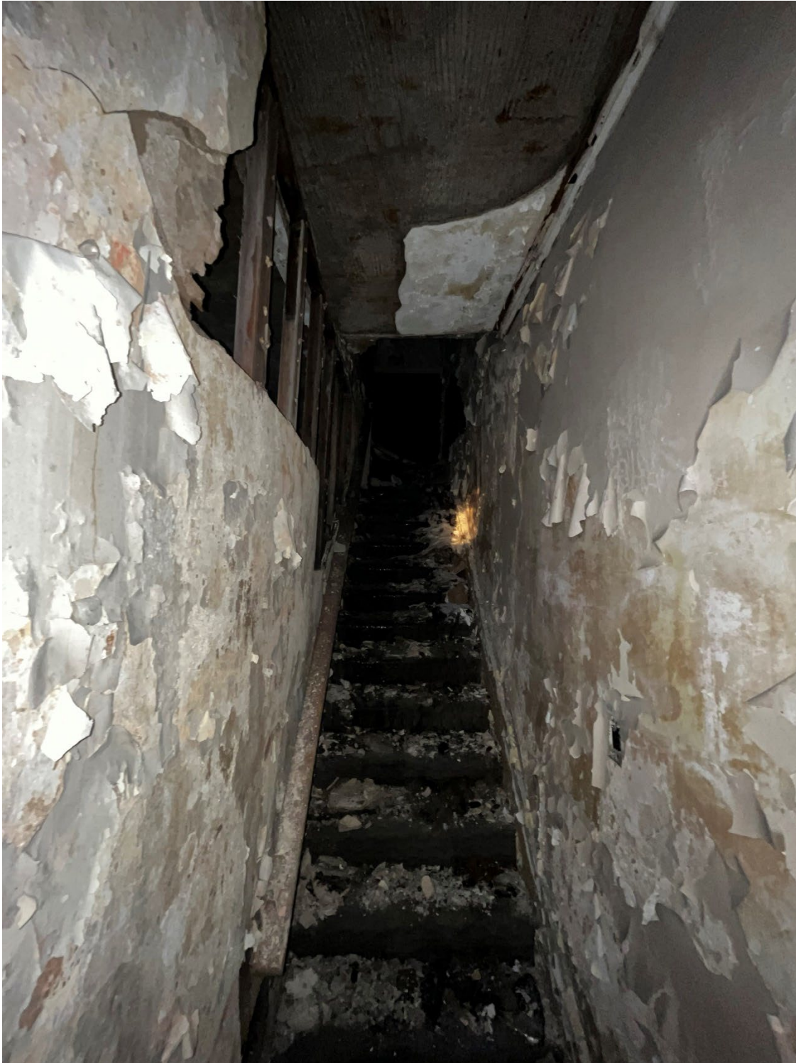
Figure 21 - Showing significant damage and staircase damaged by fire.
