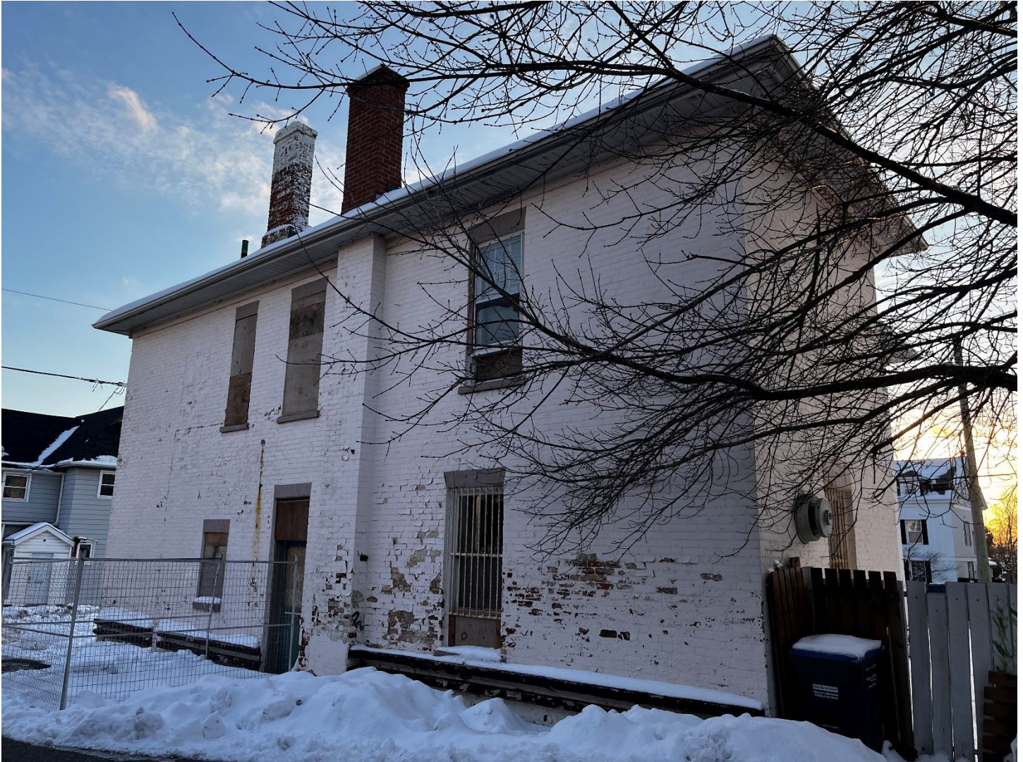
Figure 5 - Rear of building, showing damaged brick, replaced or removed original windows.
