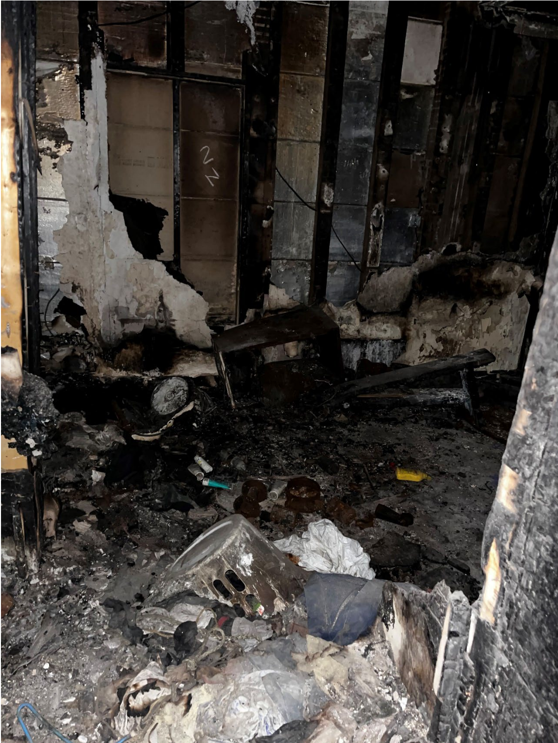
Figure 29- Showing extent of fire damage, interior black from fire and burn.
