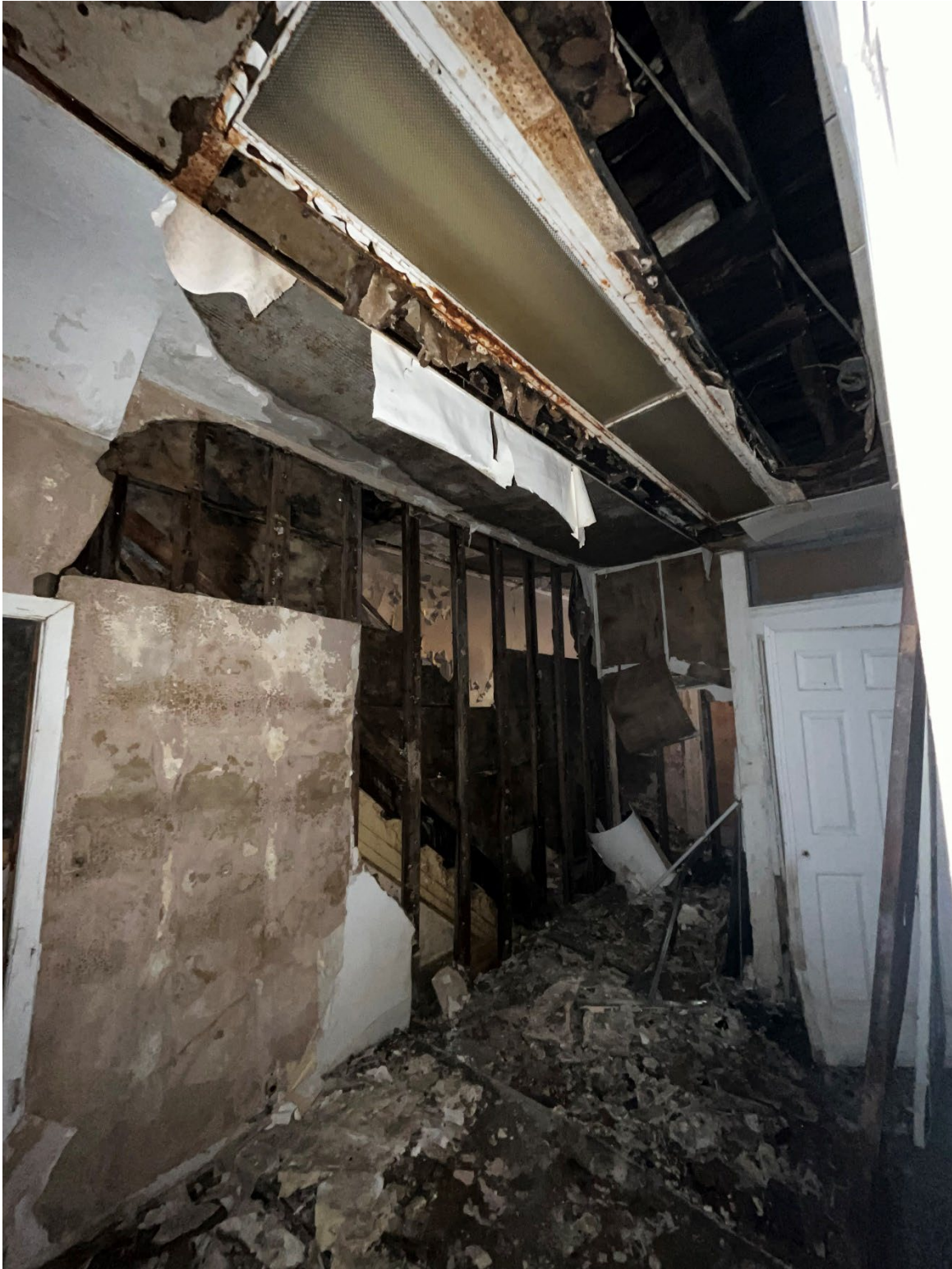
Figure 18 - Showing Significant Damage
