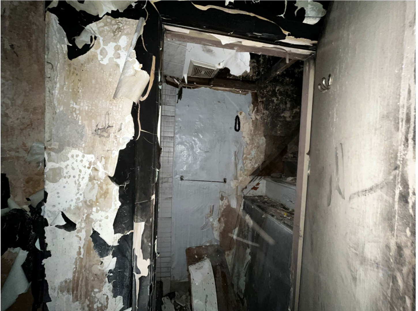
Figure 25- Showing extent of fire damage, interior black from fire and burn.
