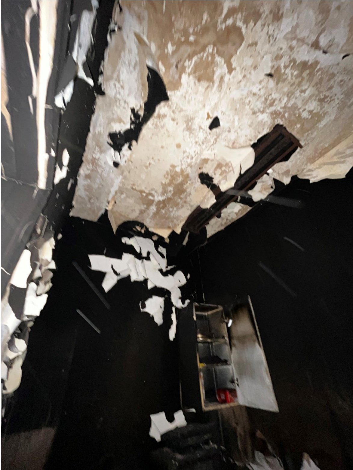
Figure 28 - Showing extent of fire damage, interior black from fire and burn.
