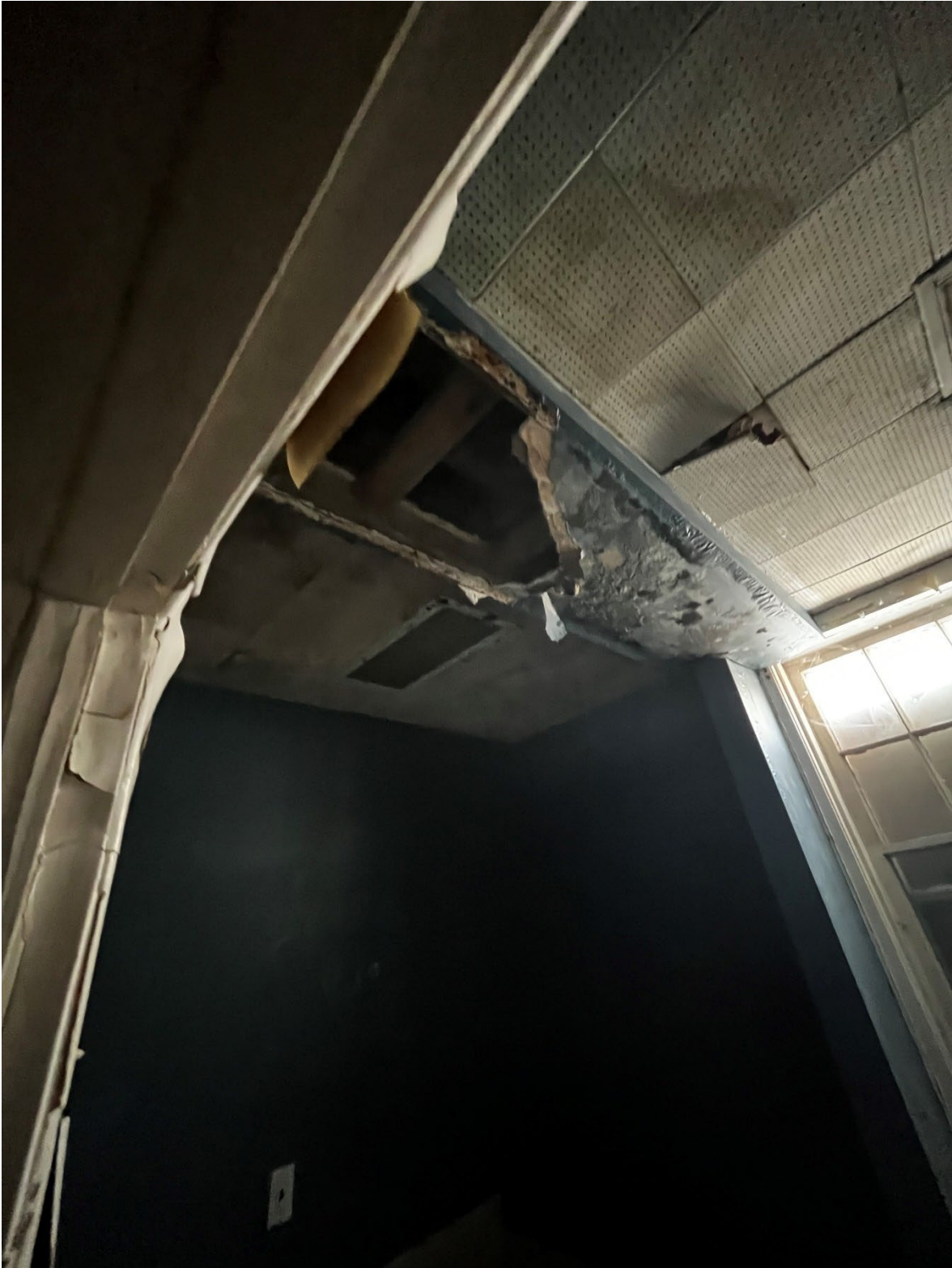
Figure 16 - Showing significant damage.
