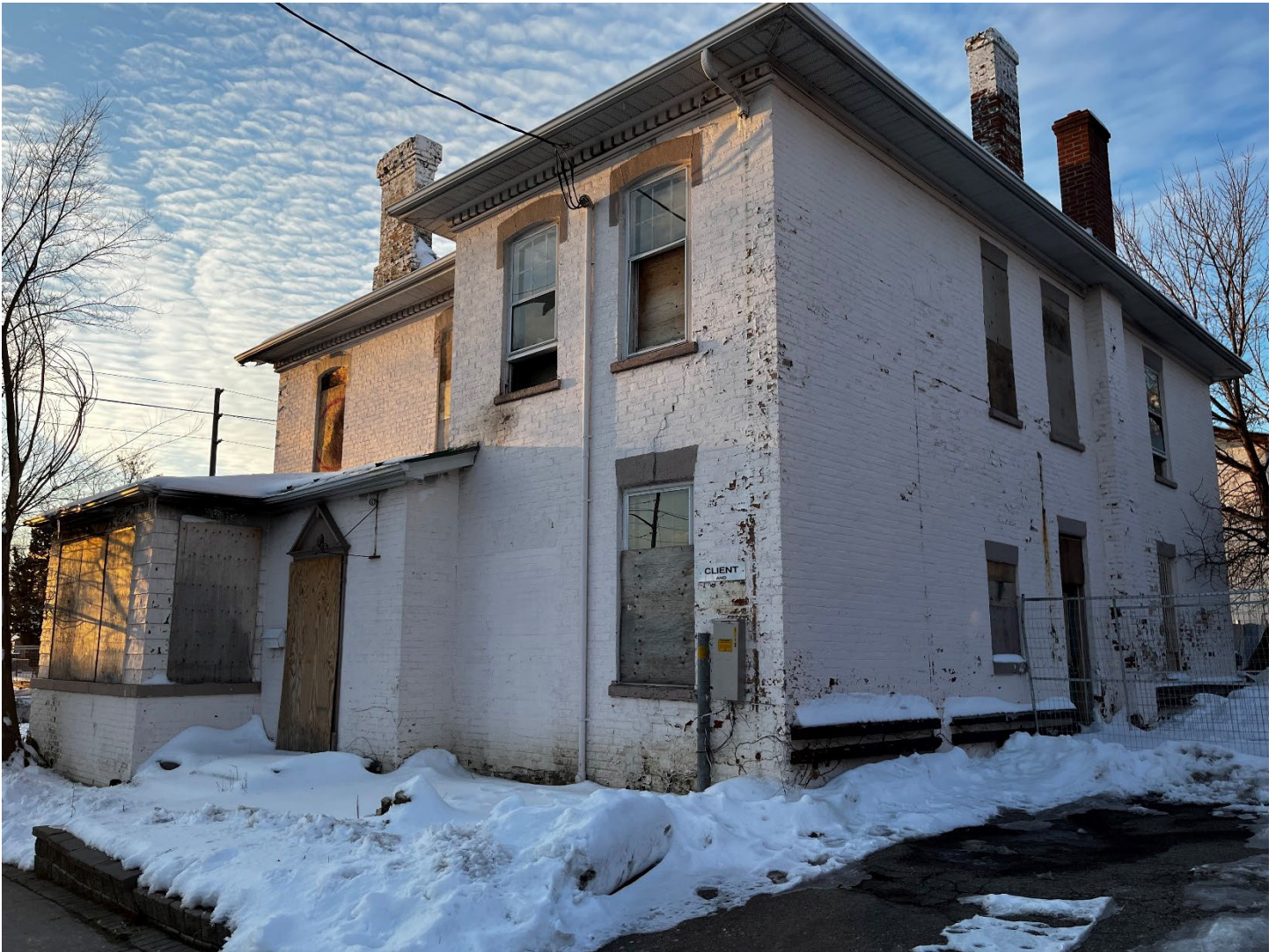
Figure 6 - Rear and South Side of building, showing deterioration of brick, replaced and removed windows, and a portion of the fire damaged section of the building. The enclosed sunroom and door was a later modification.
