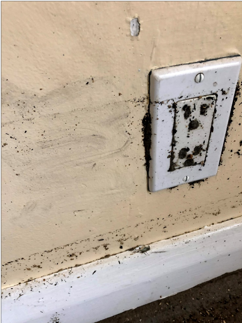
Figure 9: View of electrical socket plugged with debris
