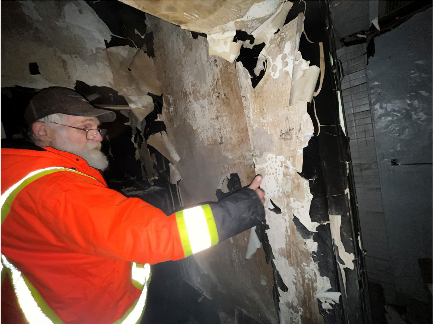
Figure 26- Showing extent of fire damage, interior black from fire and burn.
