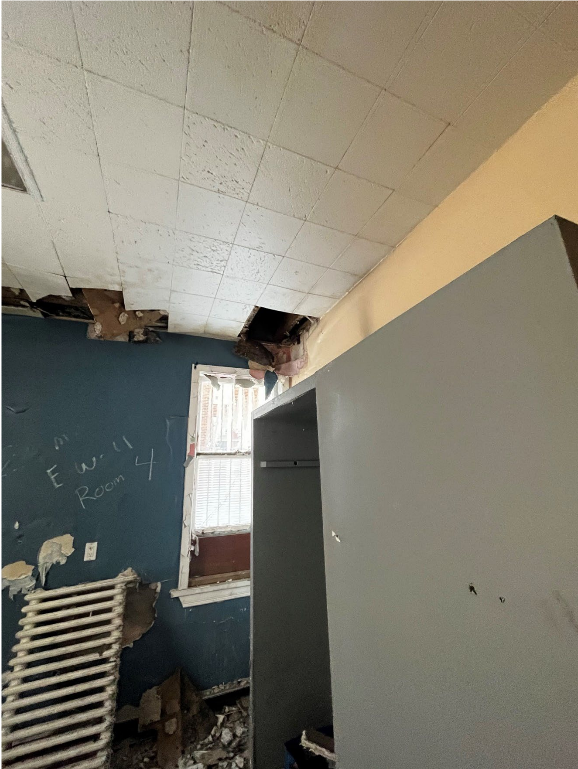
Figure 20 - Showing significant damage.
