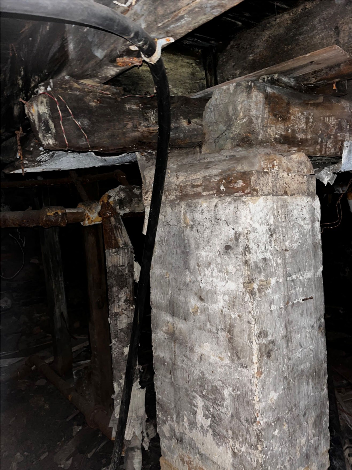
Figure 33 - Existing building foundation, with original wood beams, damaged from fire.
