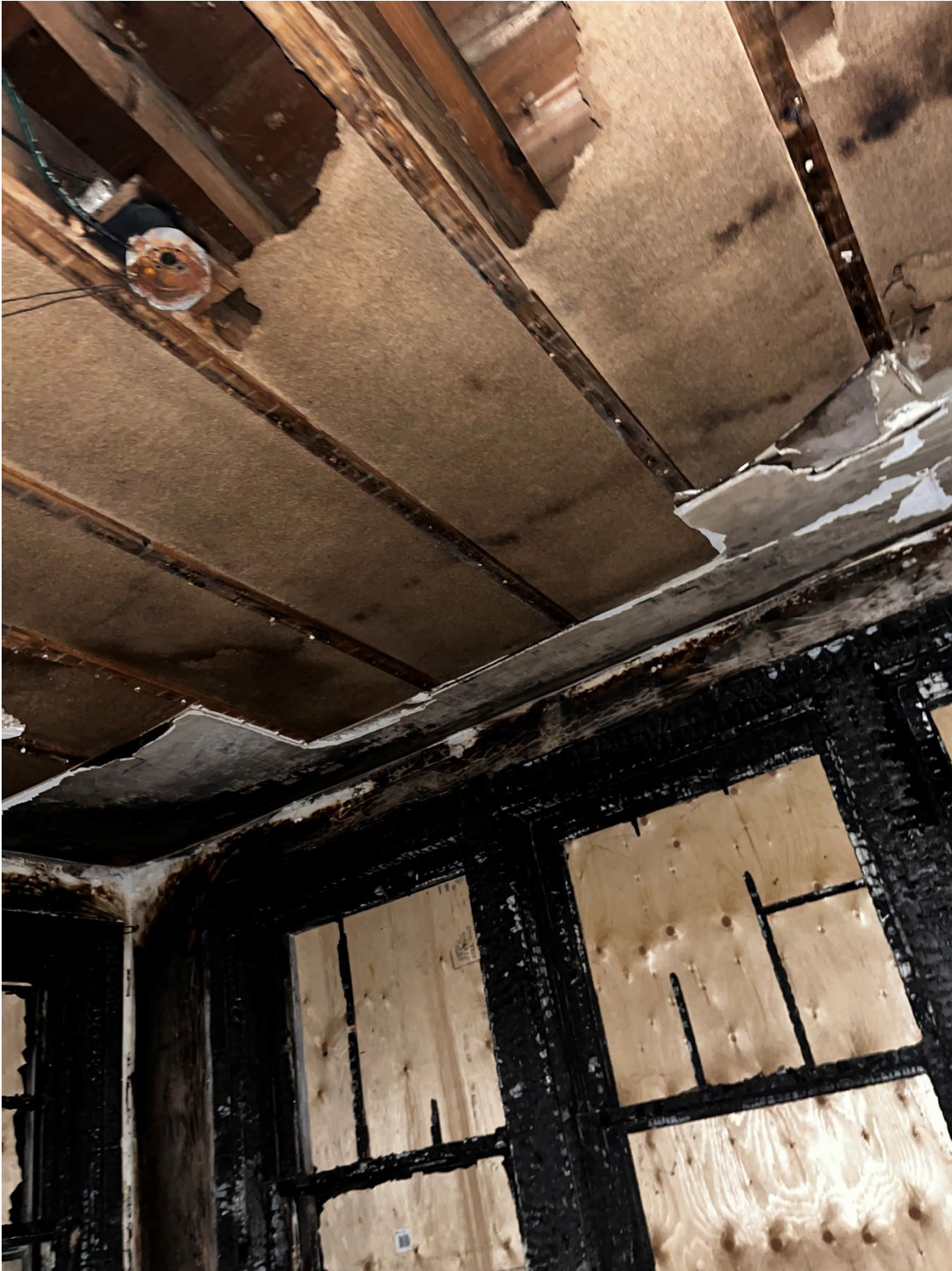
Figure 31 - Showing extent of fire damage, interior black from fire and burn.
