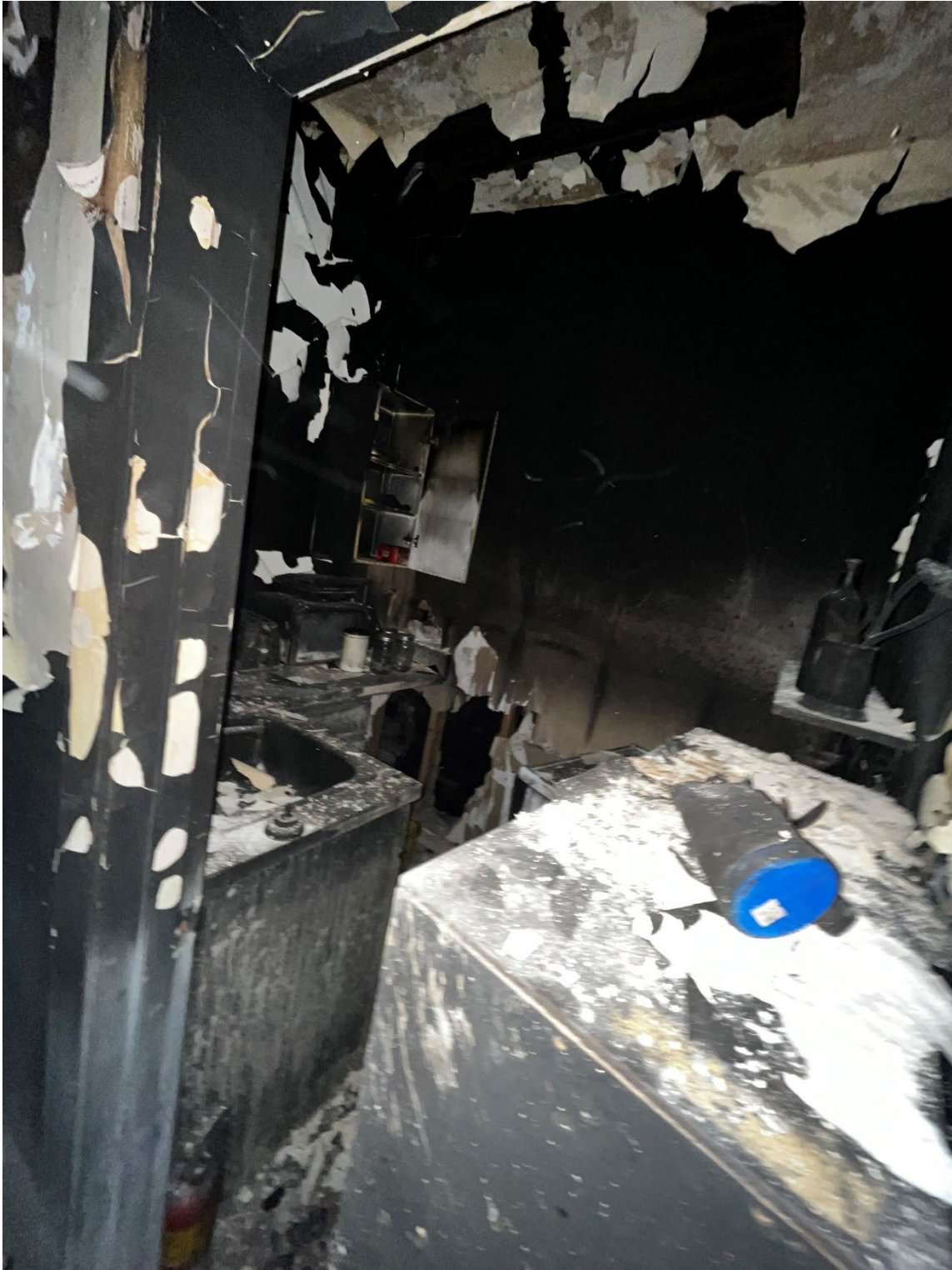
Figure 27 - Showing extent of fire damage, interior black from fire and burn.
