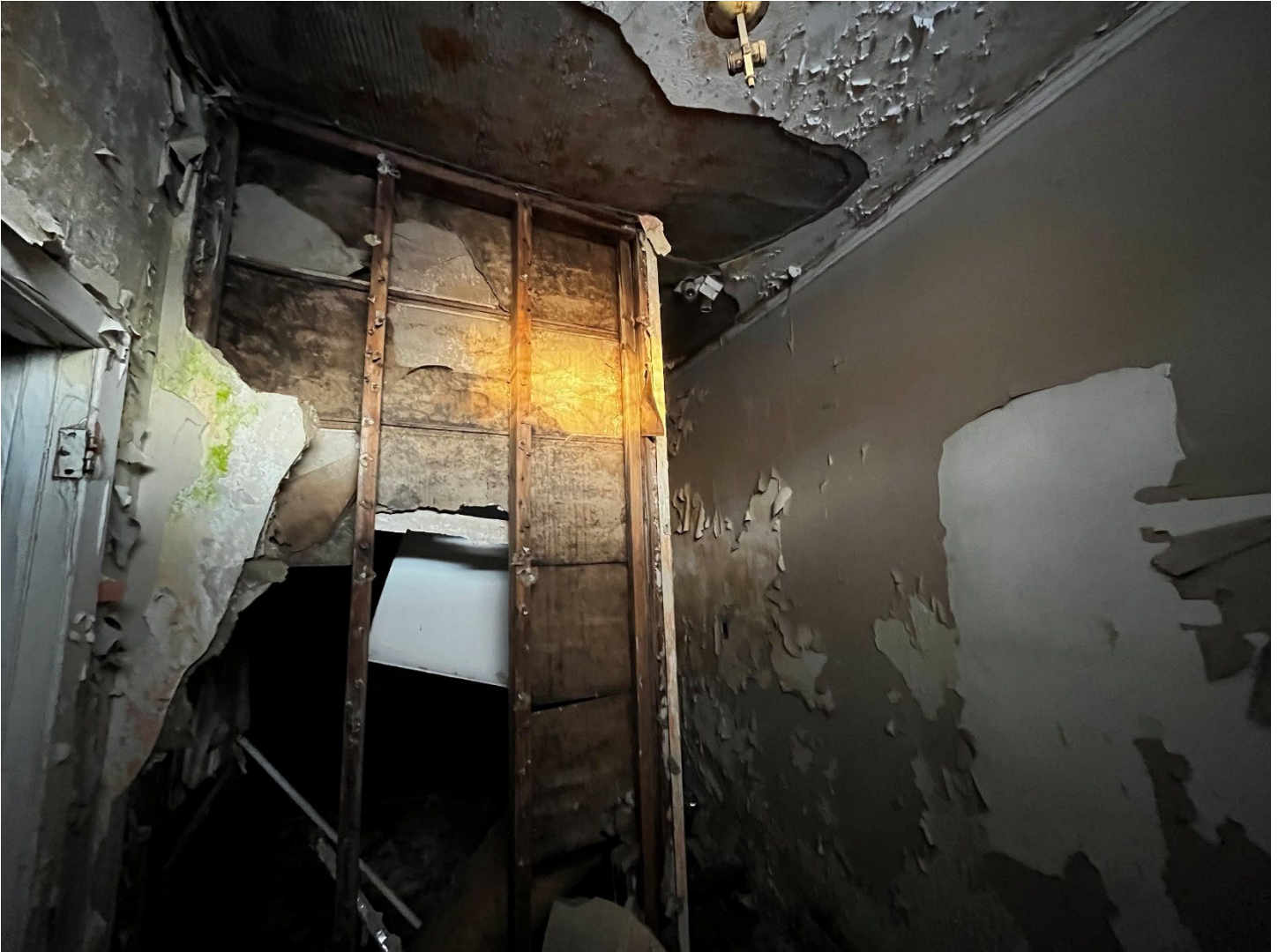
Figure 12 - Interior, showing damage.
