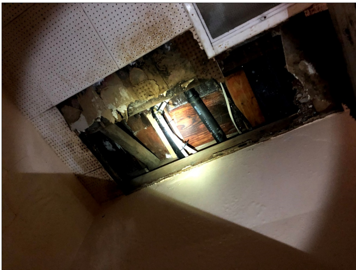
Figure 4: View of collapsing main level ceiling and water and mould damage in ceiling void
