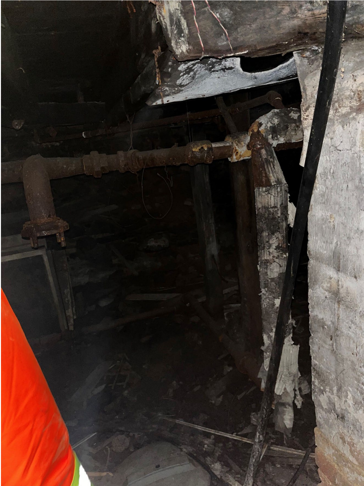
Figure 32 - Basement water system, showing damage and vandalism from arsonist.
