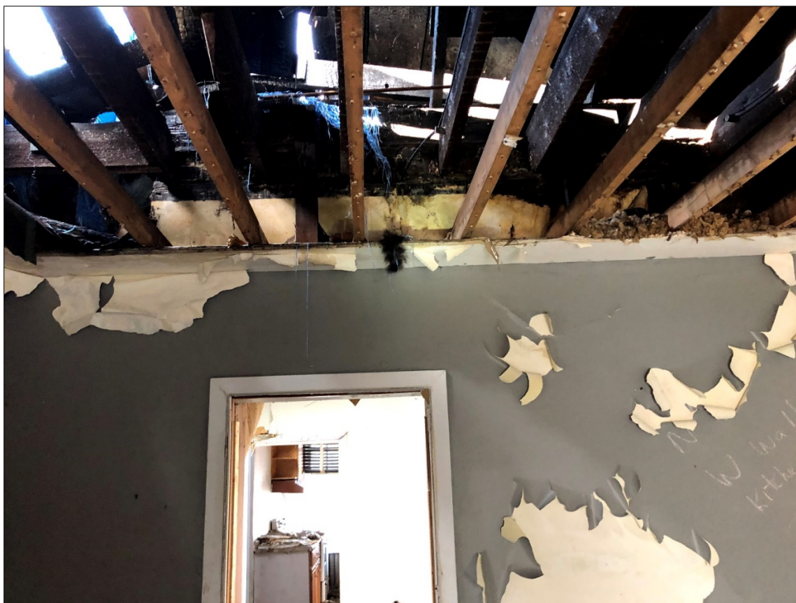
Figure 2: View of deteriorated roof and collapsed second level ceiling
