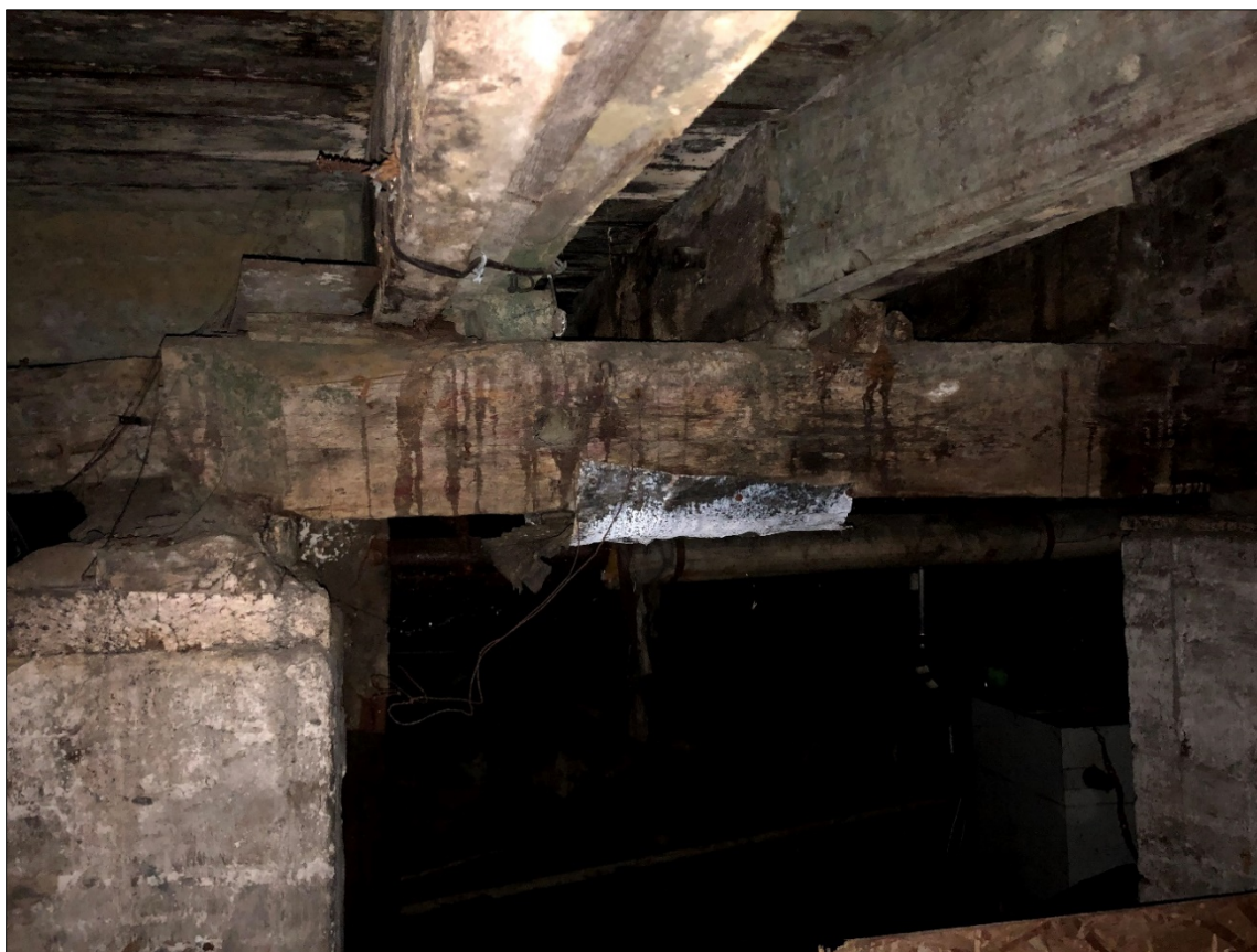
Figure 10: View of wood rot and mould impacts on basement structural members
